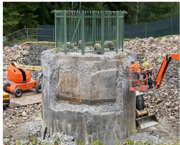
Removal of concrete collar and shotcrete exposing the octagonal concrete structure and wooden timbers
