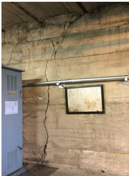
Vertical Crack in South Wall
