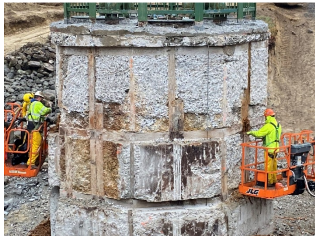
Additional vertical timbers discovered as concrete panels removed
